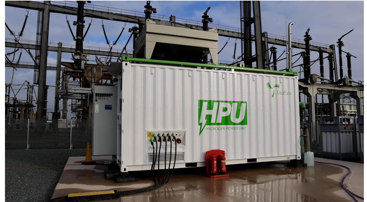
Image from National Grid ( Deeside Substation )
